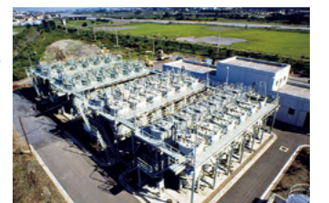
Advanced sewage treatment system
