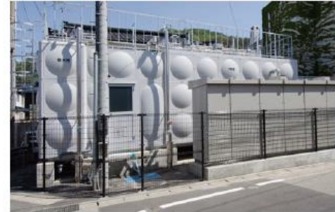
Water receiving tank and preheater
