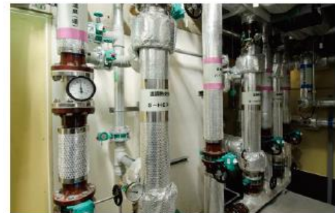
Heat exchanger chiller
